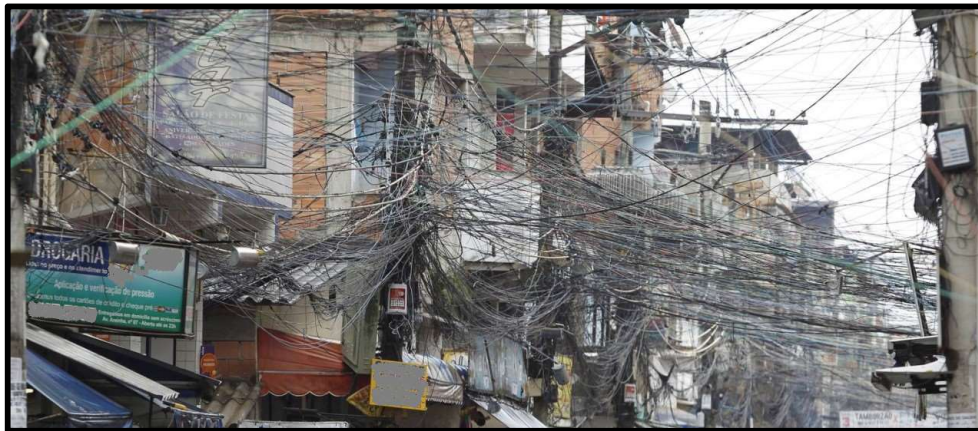
Figure 6.1 – Irregular connections in Rio de Janeiro State. Adapted from O GLOBO 26
